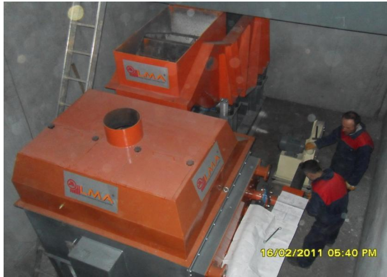
Figure-12: Mechanical reclamation system
